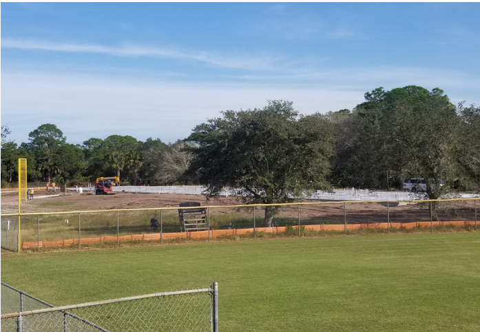
The concrete pad was poured this past week for the new CTE building as phase 1 of the new Okeechobee High School is progressing.
